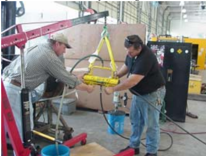
Crane riggers place the end of a wire rope into the automatic cleaning and lubrication system
